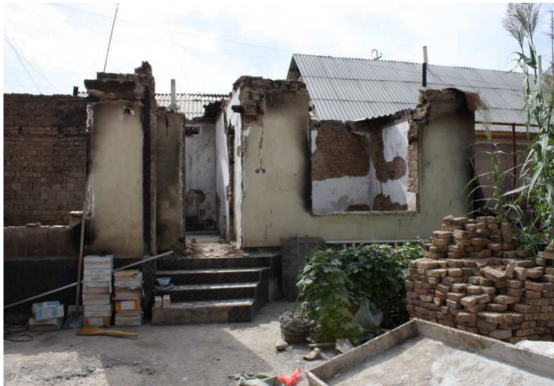
Damaged house, Jalal-Abad region
