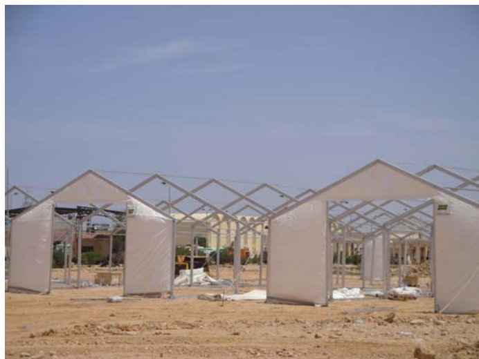
The frame of rub halls installed at the site in Saloum port. /UNHCR/N.Bose
