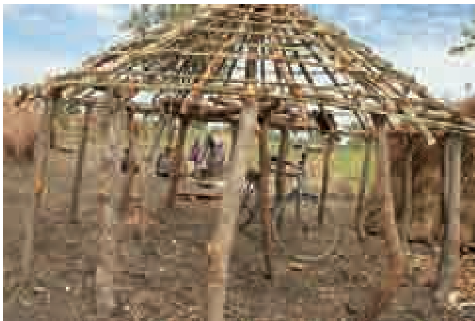
Returnees in Northern Uganda rebuilding their huts in Gulu, after years of displacement in IDP camps. UNHCR/H. Coussidis
