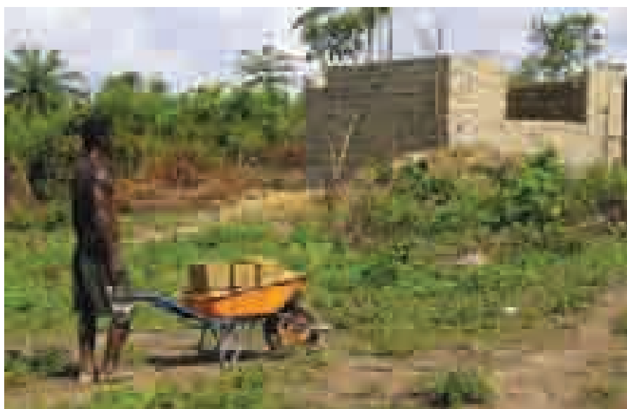
Liberia: returned IDPs. UNHCR is helping former IDPs to rebuild a school in Balama. UNHCR has been involved in a wide range of reintegration activities to help returnees, IDPs and the local community rebuild their lives. UNHCR/A.Rehrl
