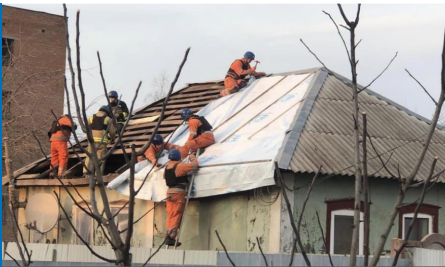
UNHCR's local partner, Proliska, provides emergency shelter support in the aftermath of shelling in Sumska oblast – 24 March 2023 © Humanitarian Mission Proliska
