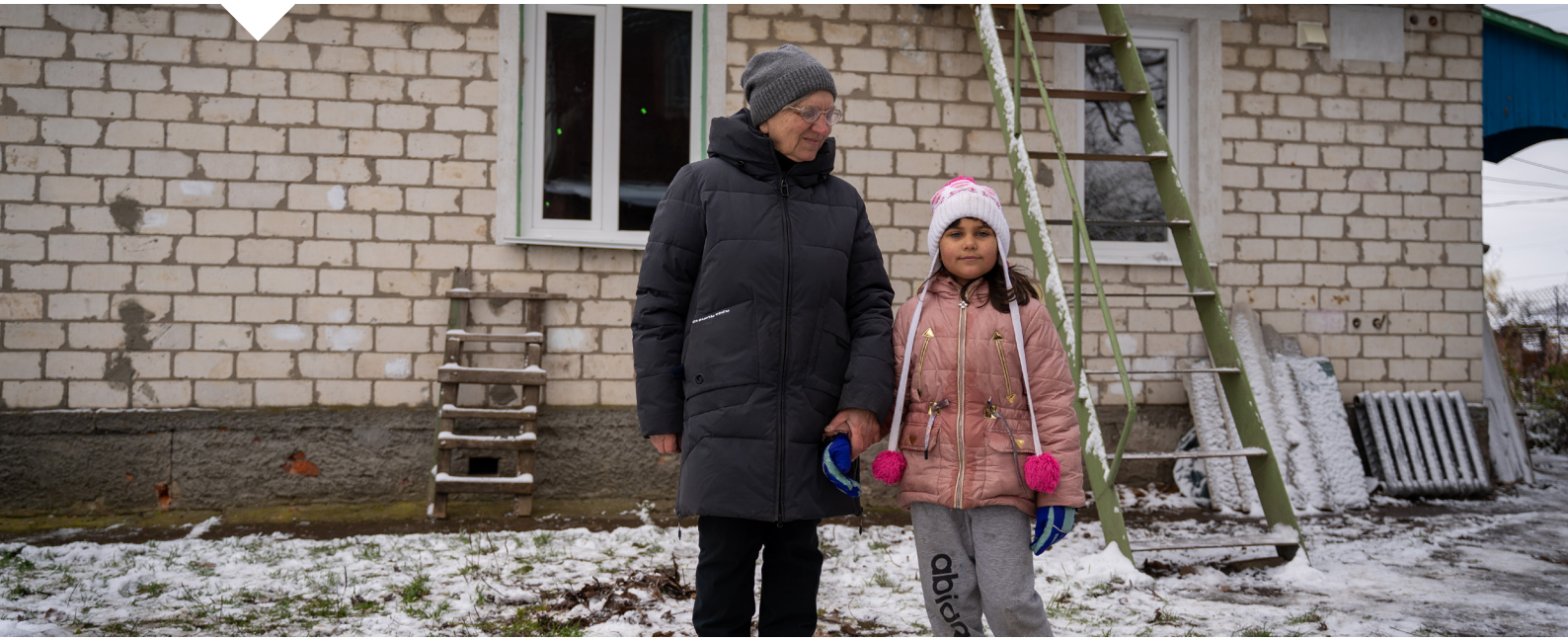
Ukraine. UNHCR supports families with house repairs so they can stay safe and warm at home, November 2022, © UNHCR/Victoria Andrievska
