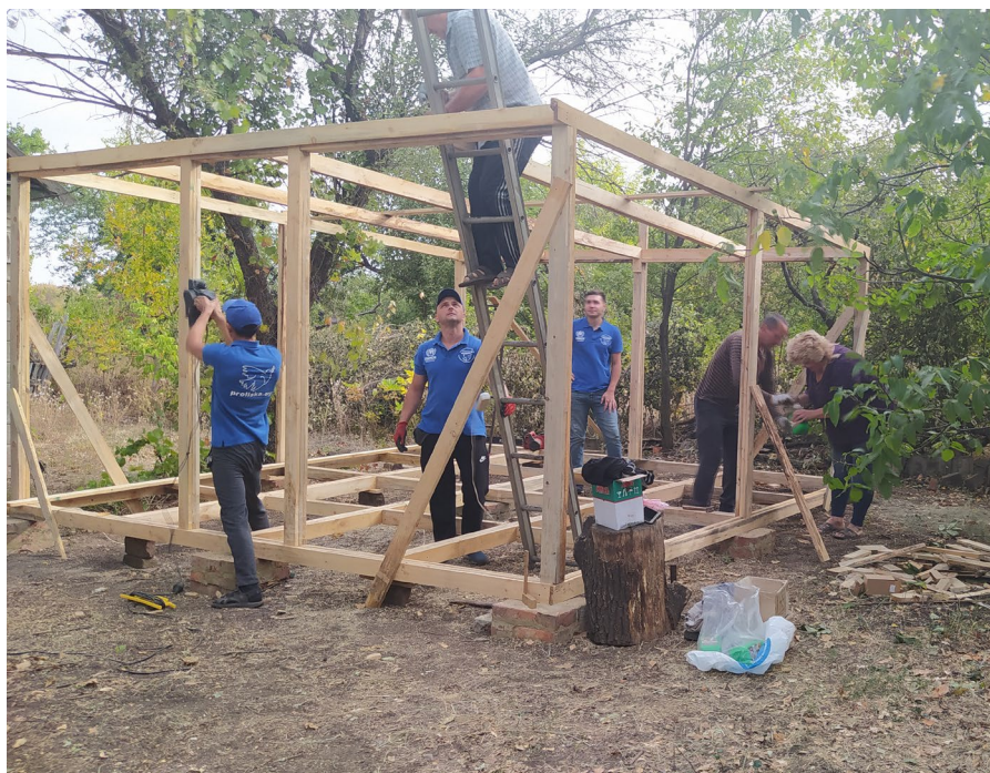
UNHCR NGO partner "Proliska" is helping to construct an outdoor terrace where local community of 105 people could hold community meetings and sessions with representatives of the NGO sector. Travneve village, Donetsk oblast, 2021 @UNHCR
