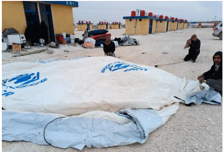
Installation of the new tents to replace damaged ones in Zone 3 in Al-Hol camp, Al-Hasakeh Governorate. ©UNHCR
