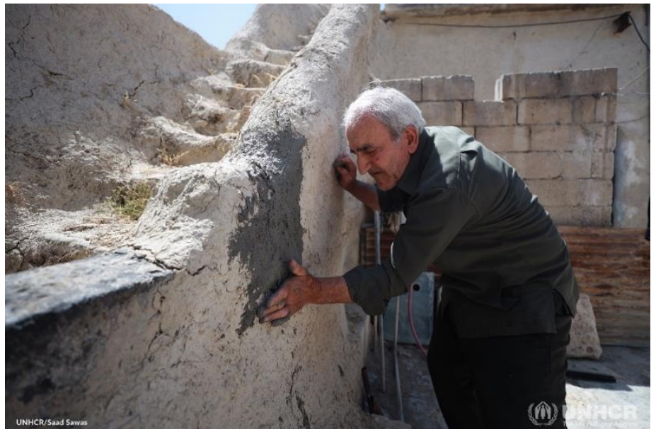
Despite the cracks that appeared on the walls of his house in rural As-Suqalabieh (Hama Governorate.) after the earthquake on 6 February, Ismail and his son had no choice but to stay. Leaving their only shelter was not an option, as they had nowhere else to go. © UNHCR/Saad Sawas
