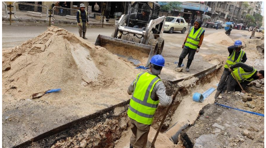
Restoration of sewage network in Sulaiman Al Halabi neighbourhood, Aleppo Governorate benefiting over 10,000 returnees. ©UNHCR/H.Maarouf
