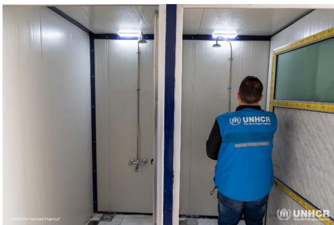
Installation of showers at a collective shelter hosting people affected by the earthquakes in Aleppo. ©UNHCR/H. Maarouf
