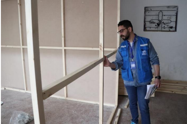
Partitions installed for added privacy at a collective shelter in Latakia. ©UNHCR/E. Kabbas
