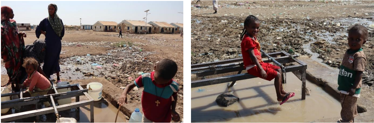
Figure 1: Water leaking at the tap stands in Shagarab's reception centre, transforming the area in a mud field; basic drainage should be implemented, beyond the direct repair.
