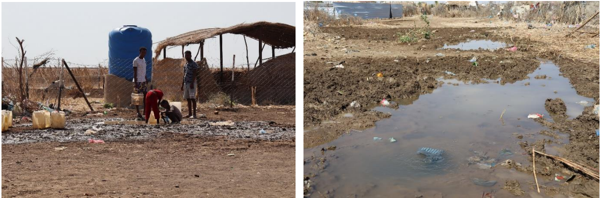
Figure 3: Left: people getting water from a pipe popping out of the ground; Right: leakage of an underground pipe.
