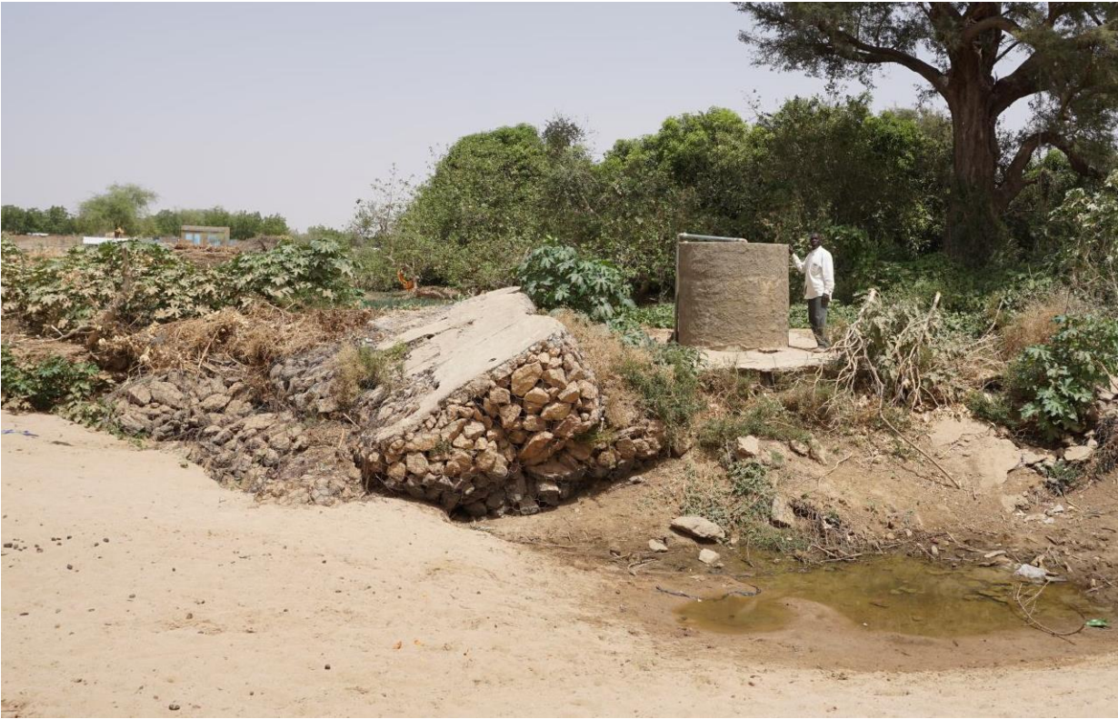
Figure 4. De-stabilization and failure of the protection works, Treguine.
