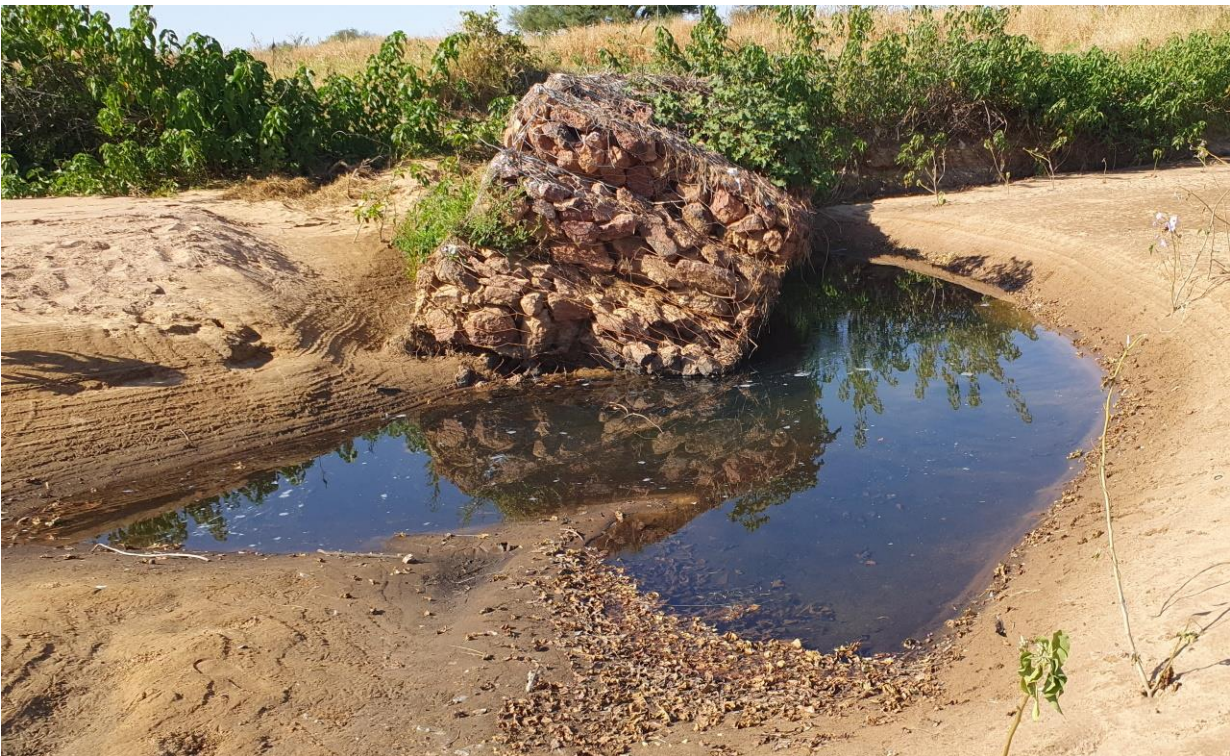
Figure 3. Scour around a gabion wall has de-stabilized it. Their lack of proper geotextile and mattress gabions as foundations meant there was no protection against scour. Durability of the cage wire is also a big concern. Hadja Hadid
