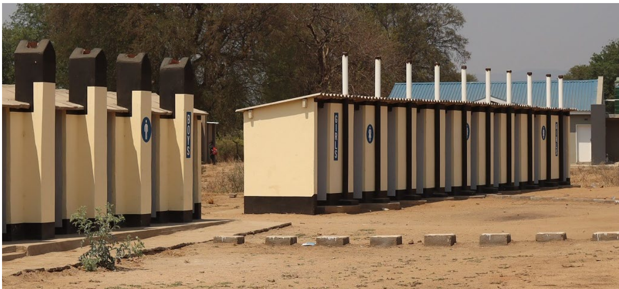
Figure 5: Vent pipes out of bricks and PVC in a school in Tongogara Refugee Camp, Zimbabwe.
