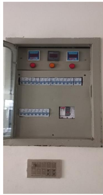
Inverter and Battery (Hall Corridor near DB of X-Ray Building)
