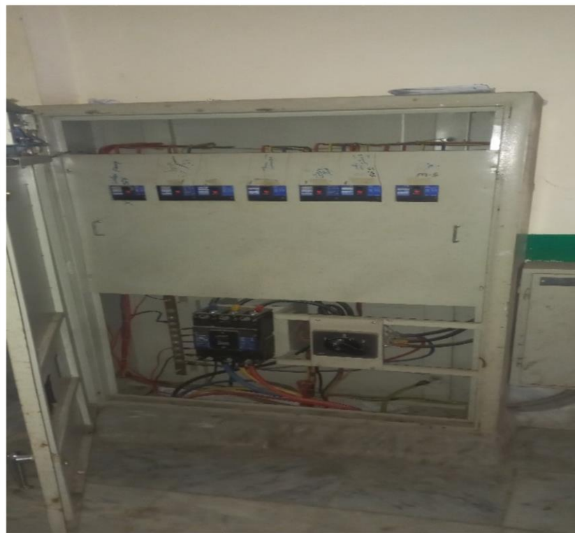
Inverter and Battery (Hall Corridor near the Main Panel)
