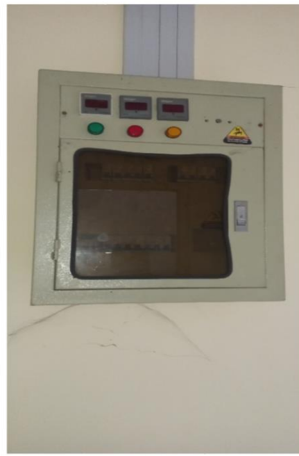
Inverter and Battery (Hall Corridor near the Main DB in Gynae Block)
