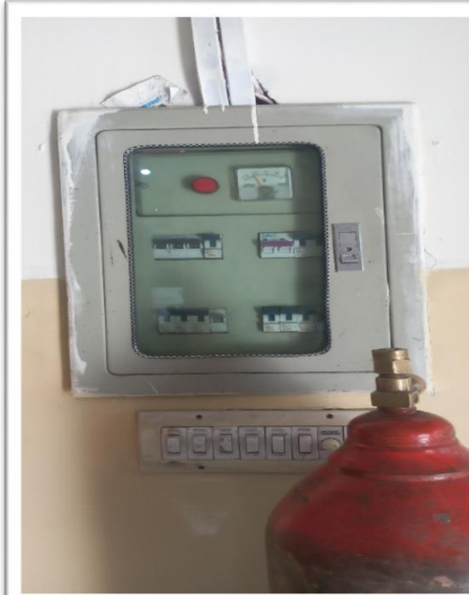
Inverter and Battery (Hall Corridor near the DB)
