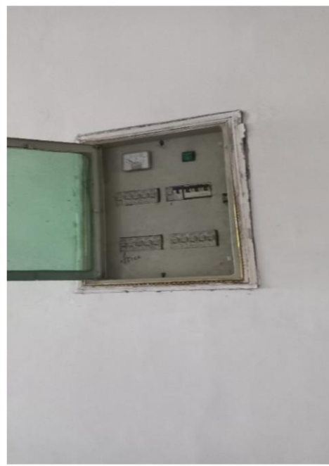
Inverter and Battery (Near the Main DB)
