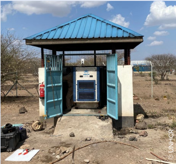
Diesel generator powering the field post in Kakuma camp
