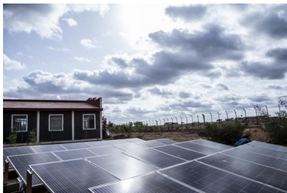
Solar technology provides reliable and constant energy to camp clinics in Melkadida. @UNHCR/Diana Diaz. 27 June 2018
