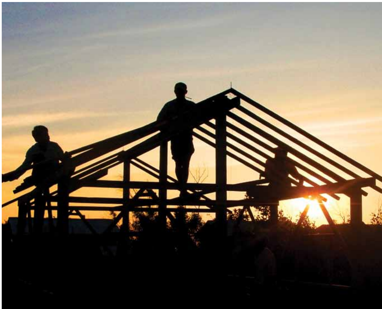
MYANMAR: Cyclone Nargis hit Myanmar in May 2008, killing 140,000 and displacing 800,000. The Norwegian Refugee Council is rebuilding homes in the hardest hit area. Diagonal beams fitted to the house frame are among the new building techniques applied, in order to make the new homes resistant to future cyclones. (Photo: Martin Suvatne/NRC)
