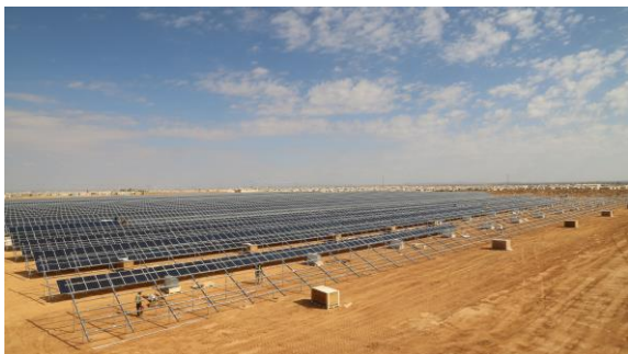
Solar panels, installed by Syrian refugees and Jordanian engineers, near completion at Za'atari refugee camp. @UNHCR/Housef Al Hariri. 12 November 2017
