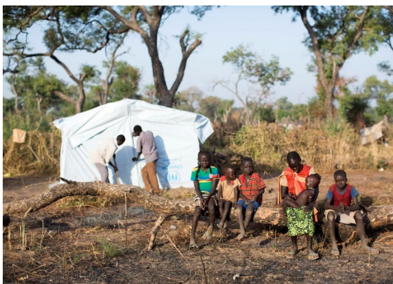
Sudanese refugees outside their new home in Ajuong Thok camp, South Sudan, as staff from UNHCR partner Danish Refugee Council fix the exterior walls. All new arrivals in Ajuong Thok are provided land and shelter materials to build their new home. UNHCR / Rocco Nuri
