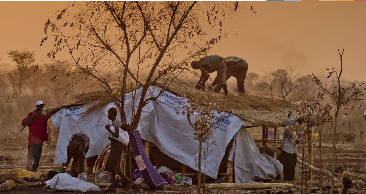
As the sun sets on Nyumanzi I settlement, many refugees are still hard at work constructing shelters. In many situations, tents, plastic sheeting and local materials available continue to be the standard. UNHCR / F. NOY / January 2014
