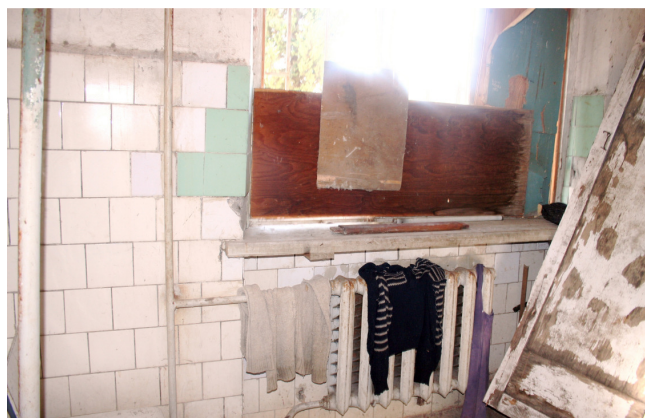
Many IDP collective centres desperately need rehabilitation work to improve living conditions
