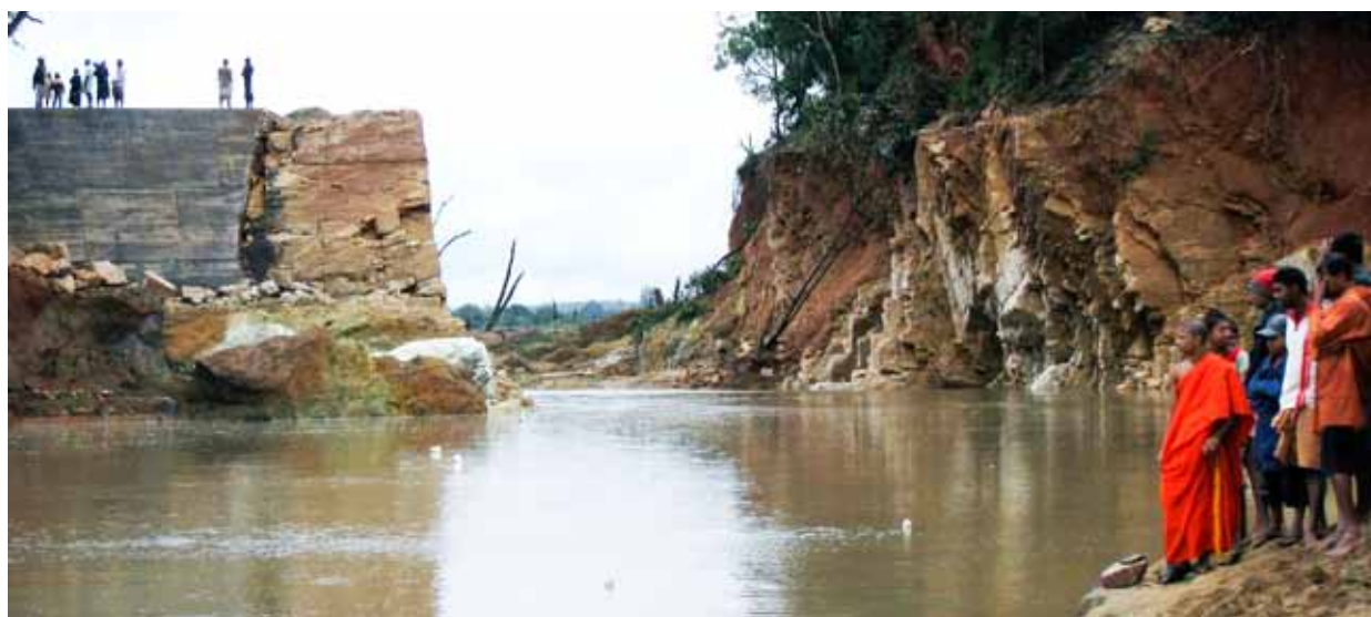
People stand near the broken walls of a large dam destroyed by flood waters in Anuradhapura district, north of Colombo, Sri Lanka, February 2011. (Photo: REUTERS/Stringer)
