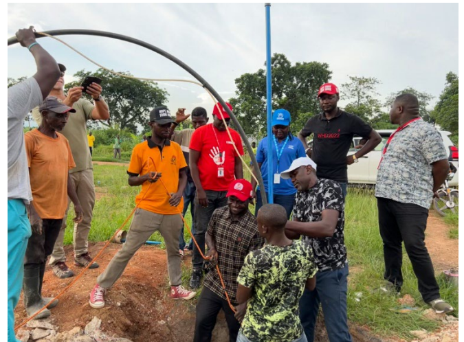
Installation of a smart water sensor inside a borehole at a refugee settlement in Ogoja-Nigeria to monitor groundwater level variation. © UNHCR
