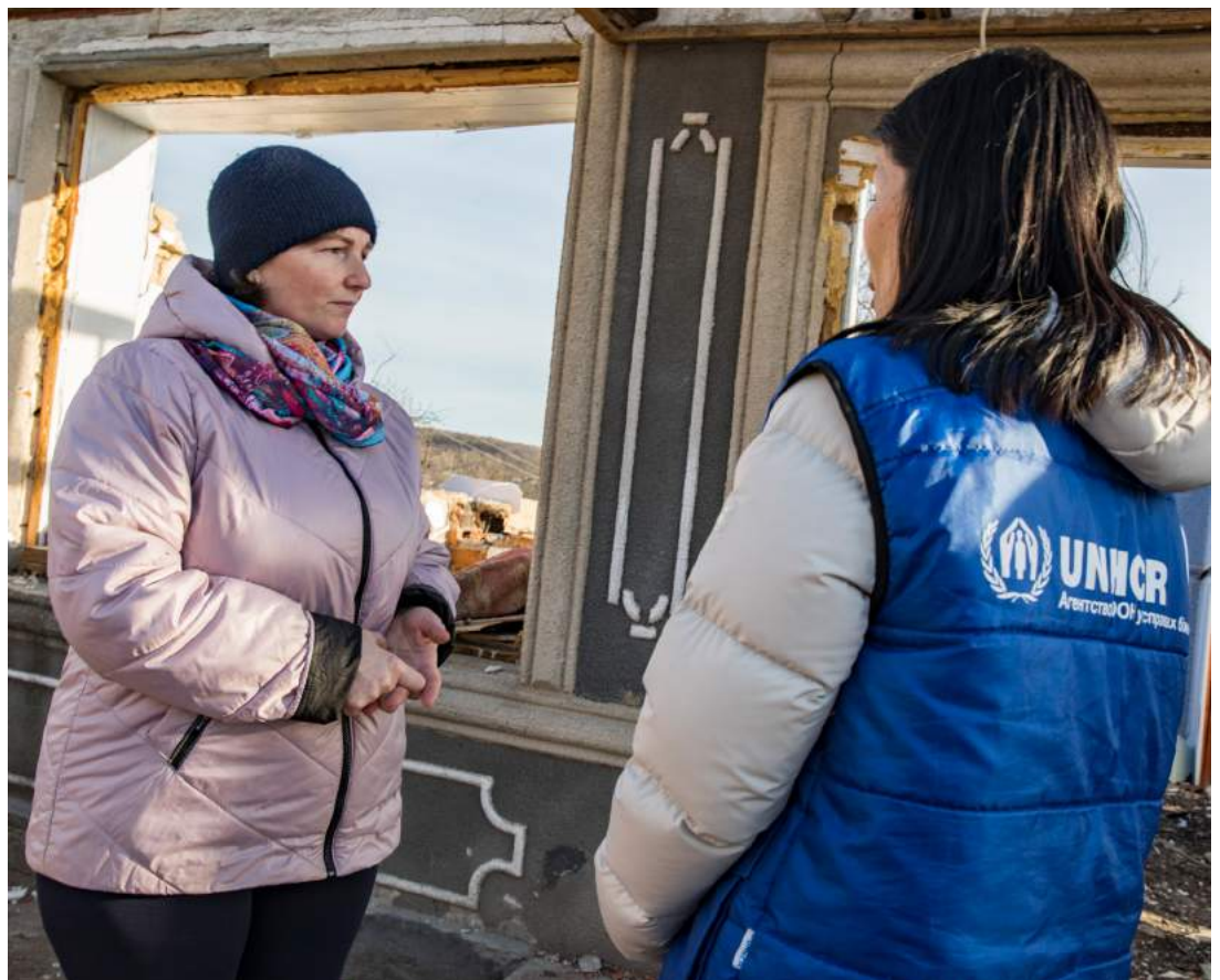
UNHCR Protection Officer Akiko Tsujisaw surveys the damage to the home of Halyna's family in a village near Tomashpil, Vinnytsia Oblast, Ukraine, following a missile attack in October 2022.
